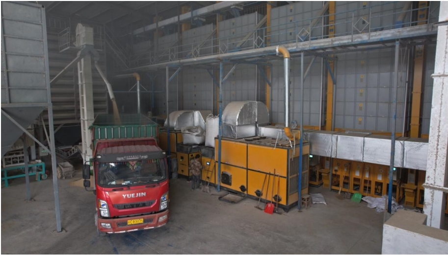
Figure 3 Grain drying line and postharvest facilities at Mashan Agricultural Service Center (Photoed by Xinfeng Ren)
